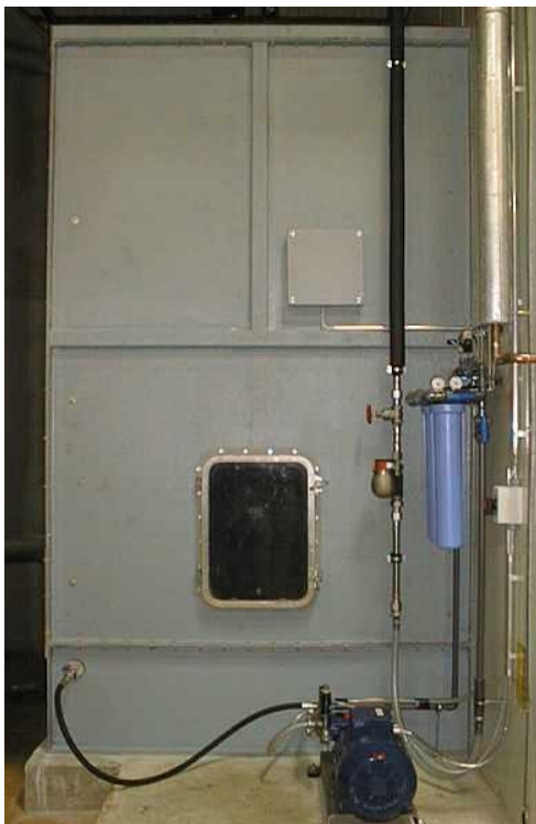
housing with pump-and filter unit
